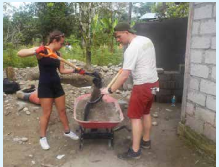
Mixing cement to construct septic tanks for the community's toilets. During our time there we built 10 toilet blocks and started construction on another 5, helped renew the local school and a number of other facilities e.g. water supply.
