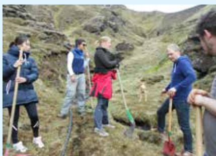
Installing the water pipe at the hikers hut in the mountains... with help from the dog! We had to put the pipe underground, and the pipe itself was fed from a mountain stream
