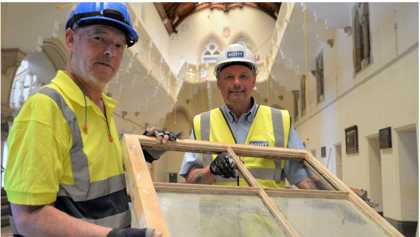
Cardigan based heritage carpenter Gary Davies (left) and Leighton Brown, Project Manager with Andrew Scott Ltd with one of the original windows from the Georgian Villas.
